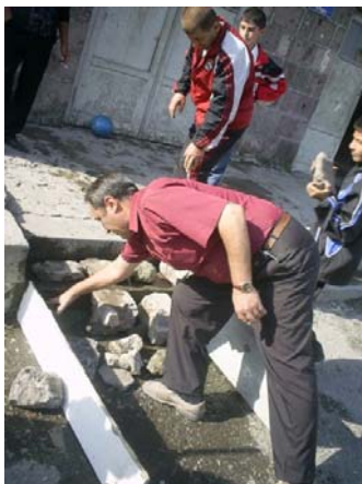
Constructing the access ramp for disabled student at Haytagh village school (Armavir Region)
